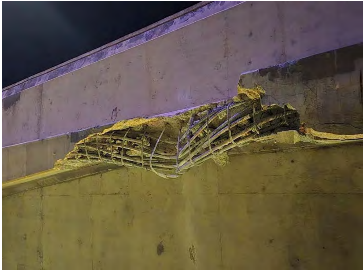
City crews are now working to repair the damaged section of the overpass (Photos courtesy City of Saskatoon)
