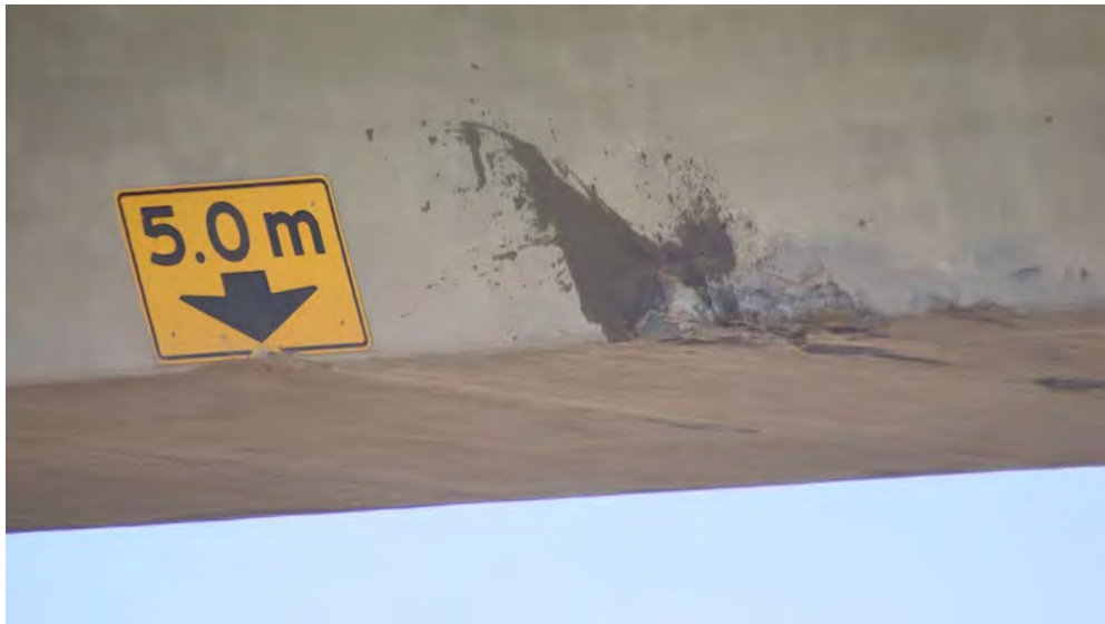
Damage underneath the railway overpass above Circle Drive is visible next to the sign indicating the clearance under the overpass is five metres. (Chanss Lagaden/CBC)
