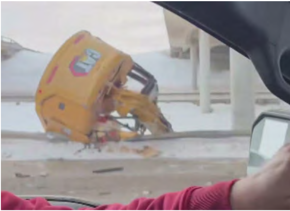
City staff don't yet have a timeline for repairs on the Circle Drive overpass. (Jacob Harmon/Facebook)
