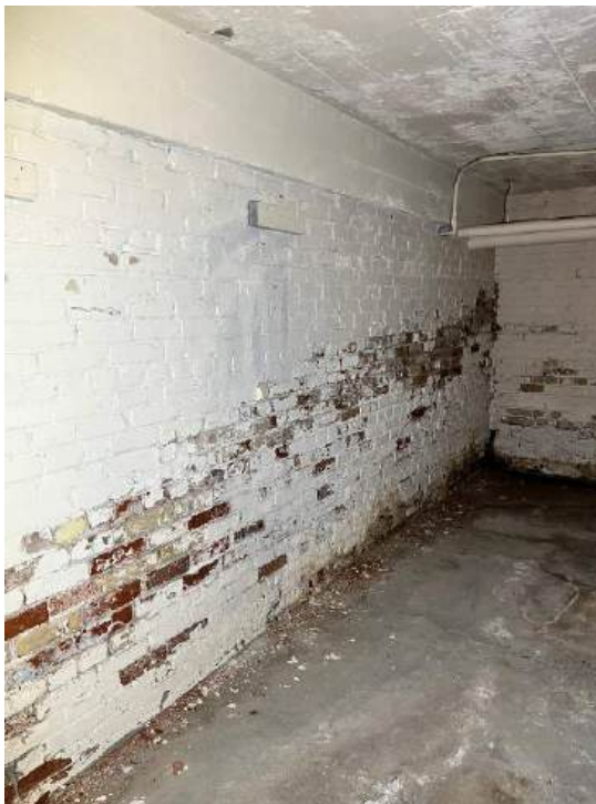
Photo 16: View of the foundation wall where moisture had caused the surface to fail
