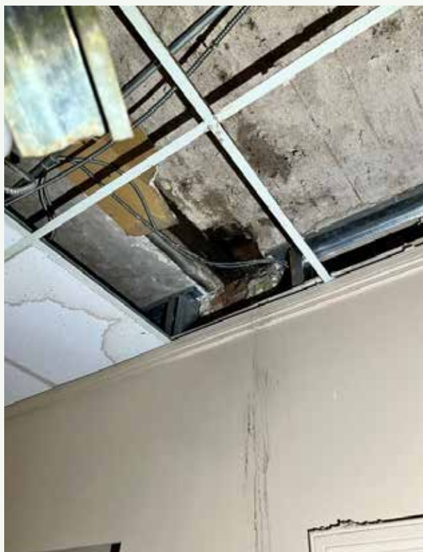
Within the wood roof structure, a metal pipe was observed where the leaks appeared to have originated.
