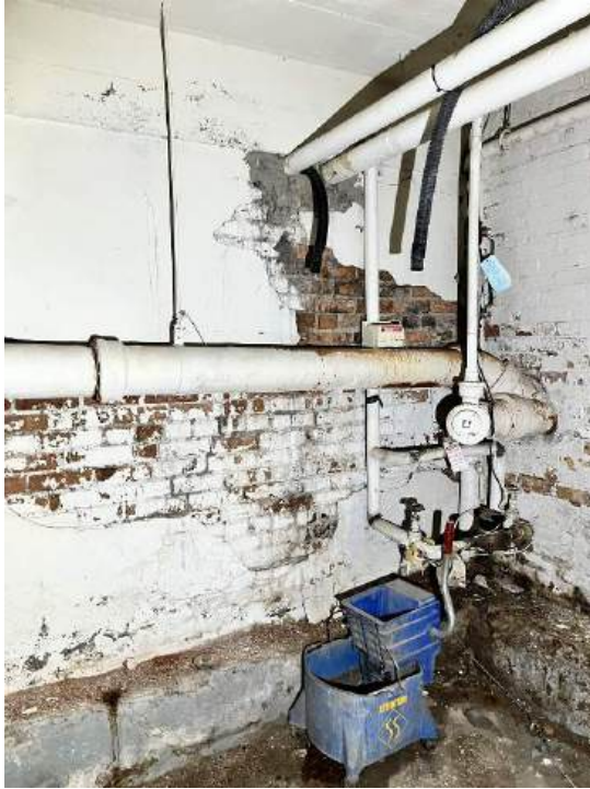
Photo 17: View of the foundation wall where moisture had caused the surface to fail
