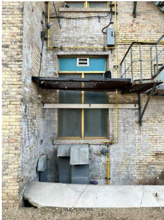
Photo 14: Uneven sidewalk above the retaining wall that had failed
