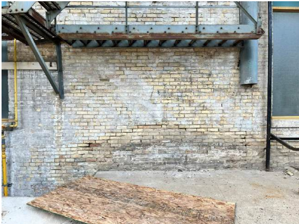
Photo 8: Eroded mortar joints on the east elevation
