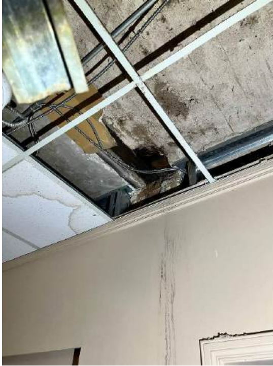
Photo 24: Within the wood roof structure, a metal pipe was observed where the leaks appeared to have originated.
