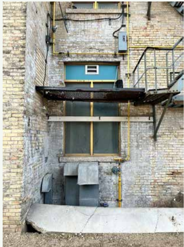
Uneven sidewalk above the retaining wall that had failed
