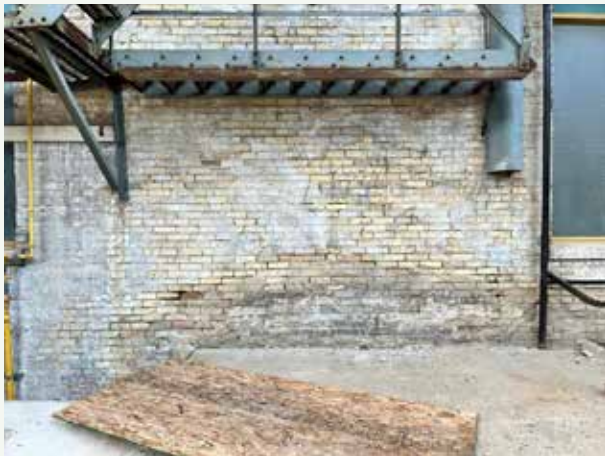
Eroded mortar joints on the east elevation
