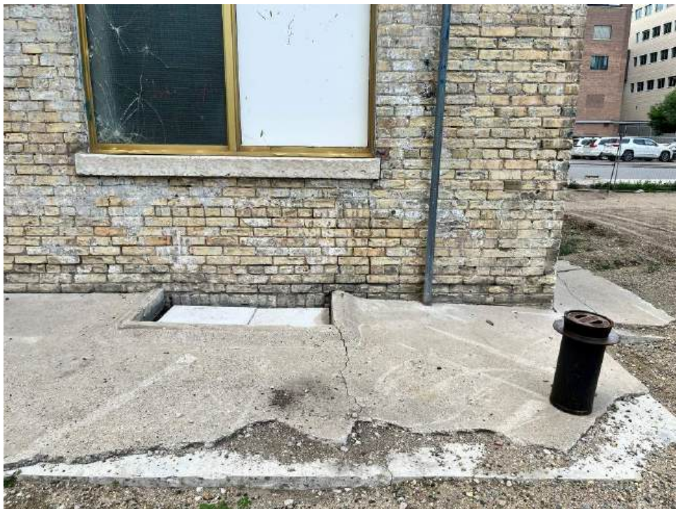
Photo 10: Eroded mortar joints, deteriorated brick masonry, and cracks from differential movement
