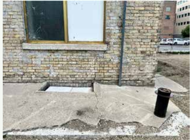
Eroded mortar joints, deteriorated brick masonry, and cracks from differential movement
