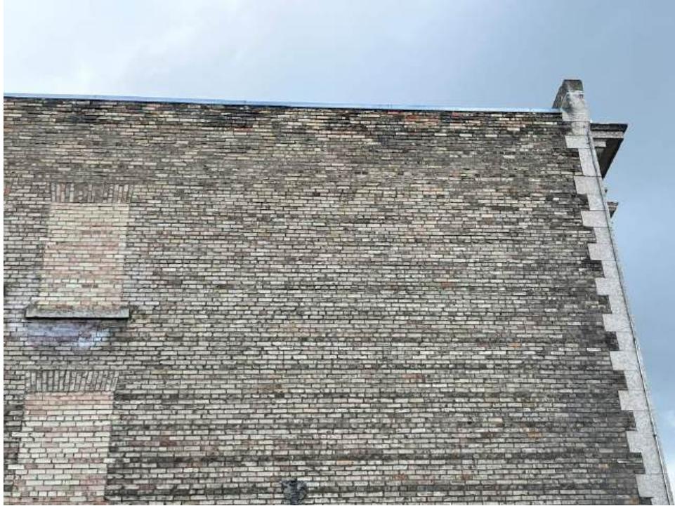
Photo 13: Partial elevation of the north side of the building where mortar joints have eroded at the parapet
