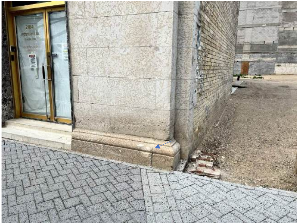
Photo 4: Cracks observed in the mortar joints and discoloration of the stone from moisture
