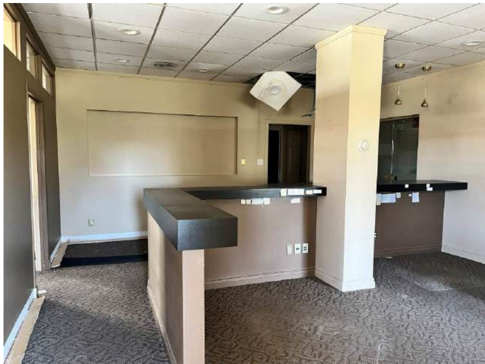
Photo 23: View of the Third Floor, also showing the location of the water leak
