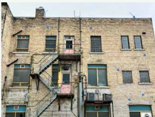
Cracks observed throughout the wall and eroded mortar joints at the parapet
