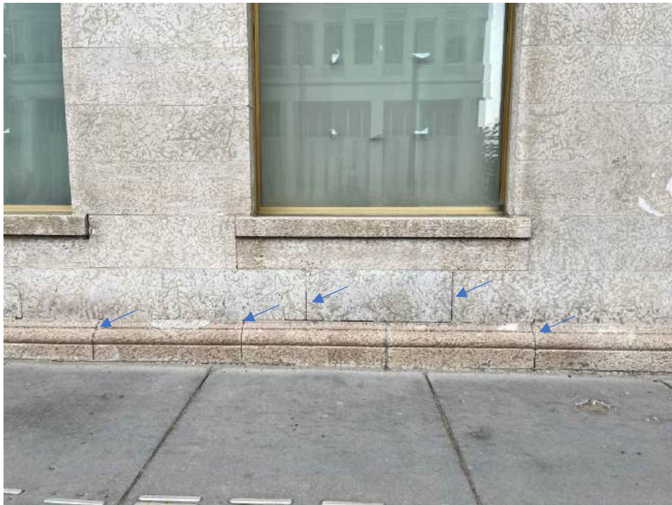
Photo 2: Cracks observed in the mortar joints and stones on the west elevation
