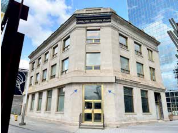
Cracks observed in the mortar joints and stones on the west elevation.
