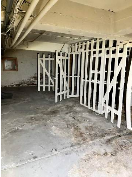
Photo 15: Heaved floor slab in the basement with cracks and efflorescence. Typical slab and beam construction could also be observed in the basement.
