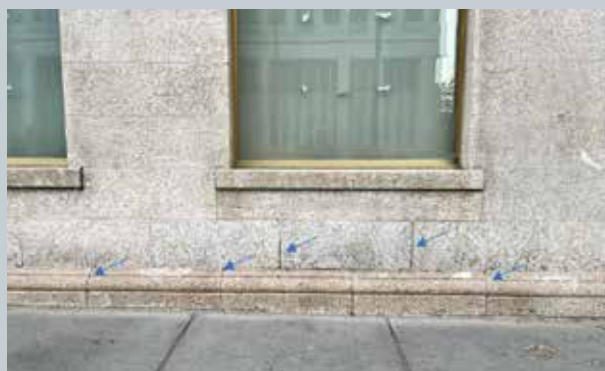
Cracks observed in the mortar joints and stones on the west elevation.
