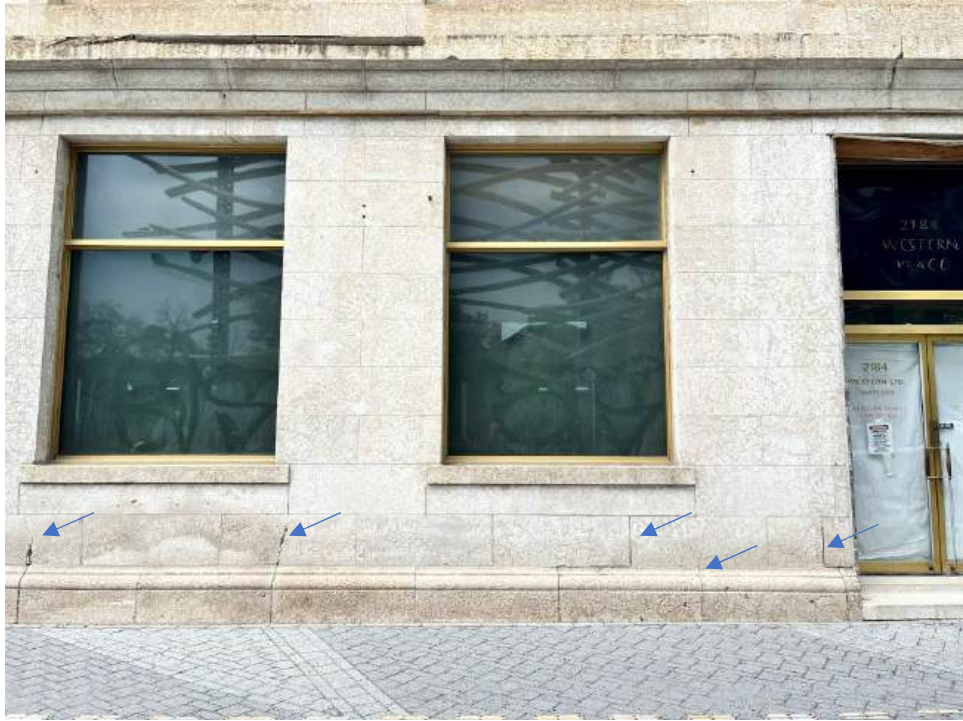
Photo 3: Cracks observed in the mortar joints and stones on the south elevation
