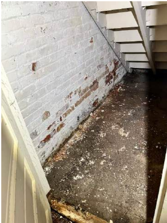
Photo 18: View of the foundation wall where moisture had caused the surface to fail
