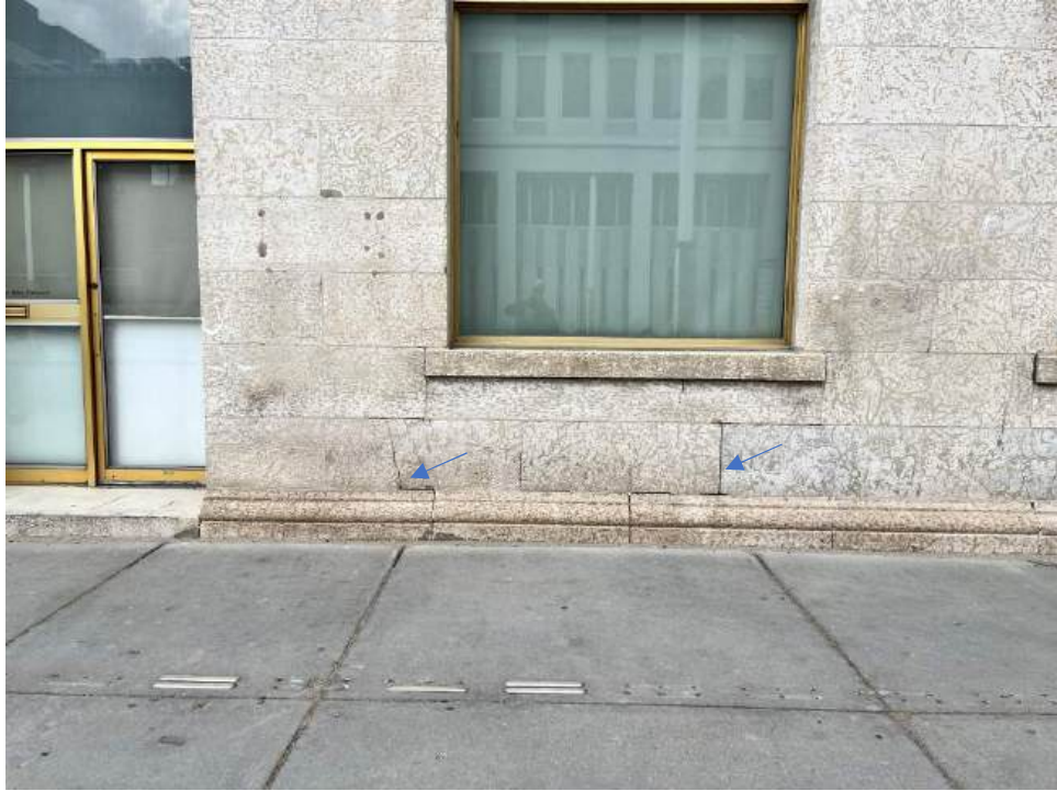
Photo 1: Cracks observed in the mortar joints and stones on the west elevation
