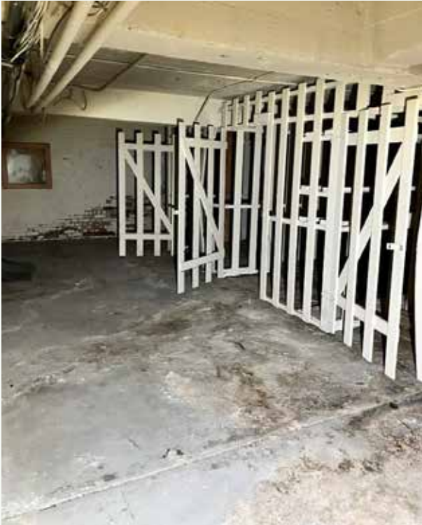
Heaved floor slab in the basement with cracks and efflorescence.
