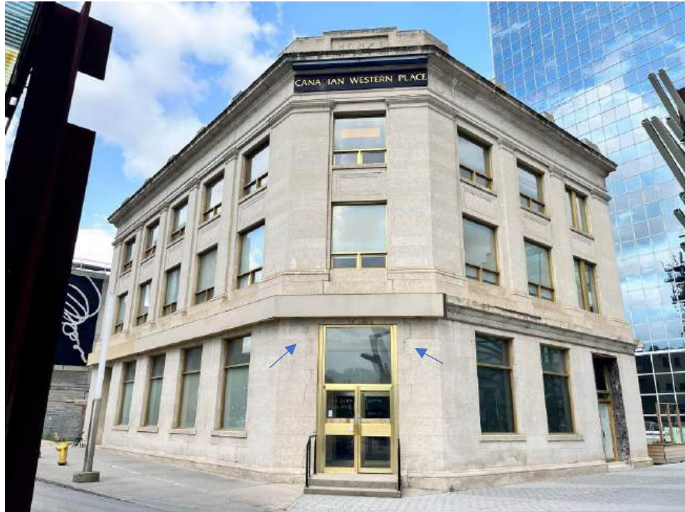
Photo 5: Cracks in the mortar joints around the southwest entrance
