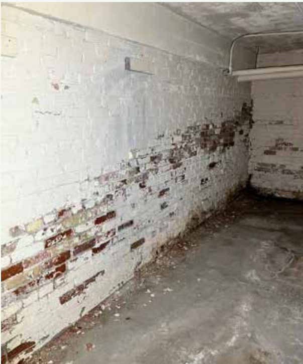
View of the foundation wall where moisture had caused the surface to fail
