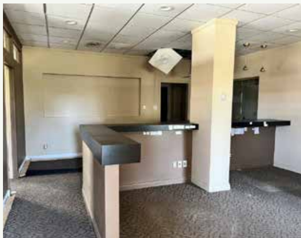
View of the Third Floor, also showing the location of the water leak
