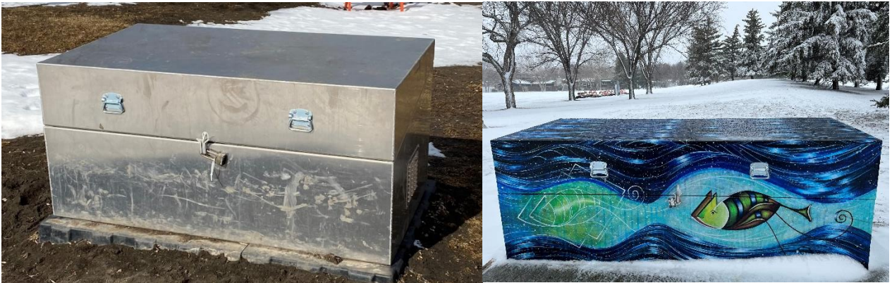
Example of Water Service Box
